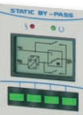
Display static bypass
